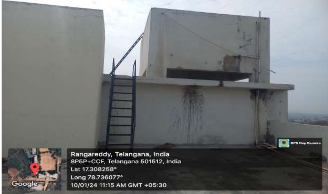
Overhead tank at AITH (B-Block)
