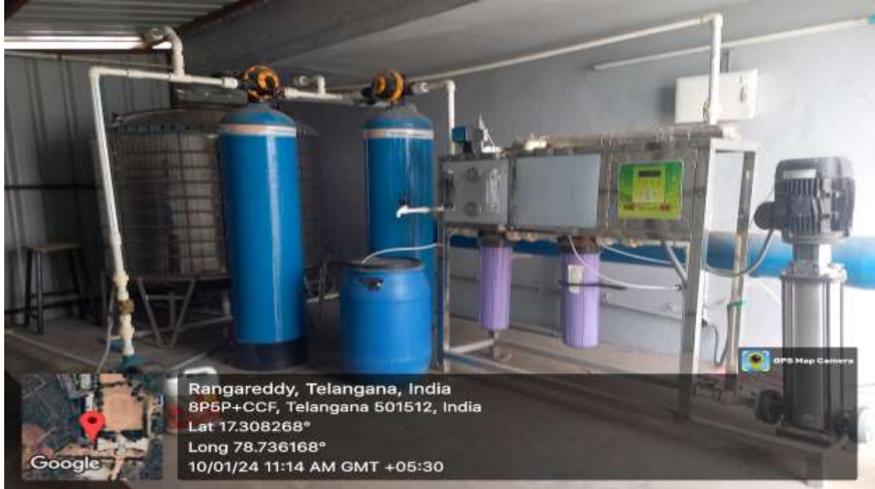
RO plant in Campus
