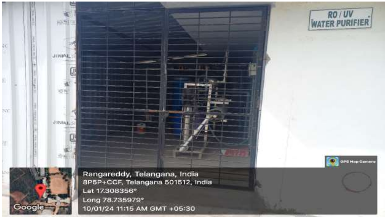
RO plant in Campus
