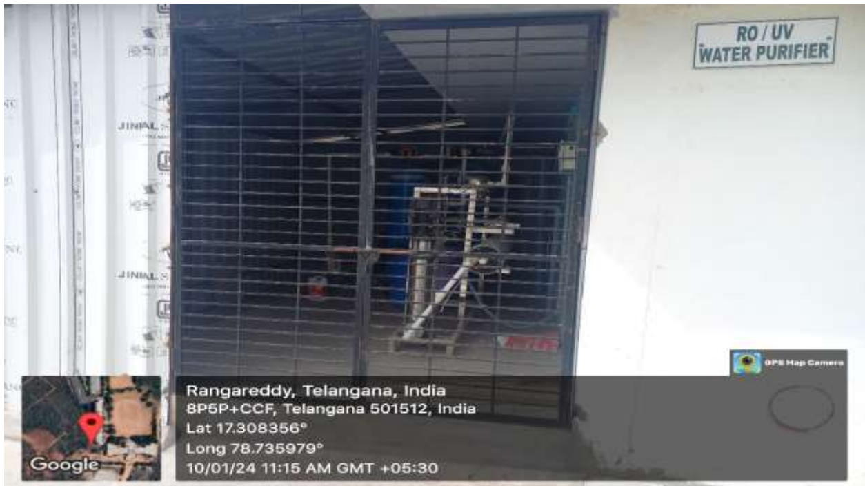
R O plant installed in A and B Blocks
