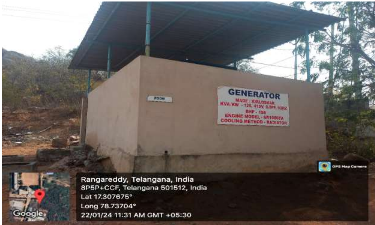
Generator Room at AITH
