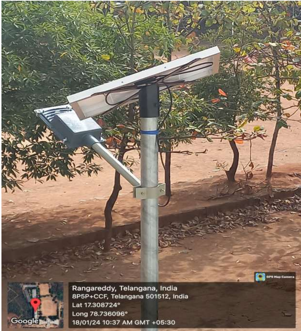
Solar Light at AITH
