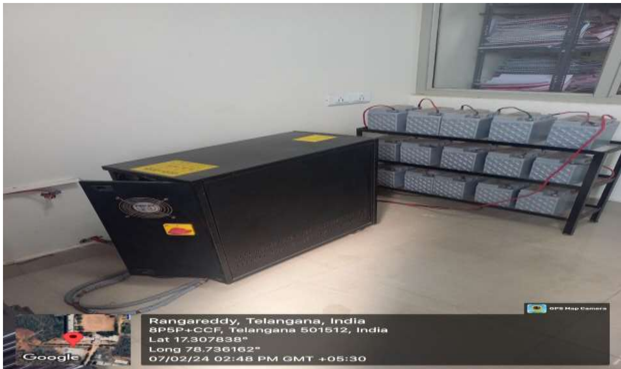
UPS / Inverter at AITH
